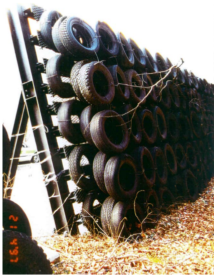
Fig. 3: Rockfall barrier built of steel beams and old tires at Matsubarako, Nagano Pref., Japan.
