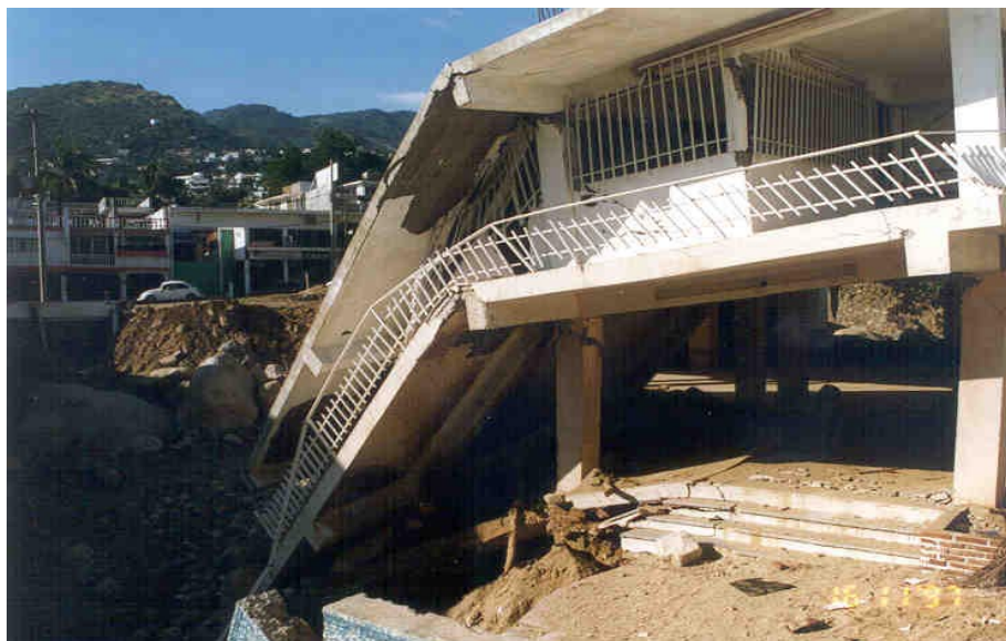
Figure 5. Building devastated and partly collapsed after foundation undercut by torrent.
