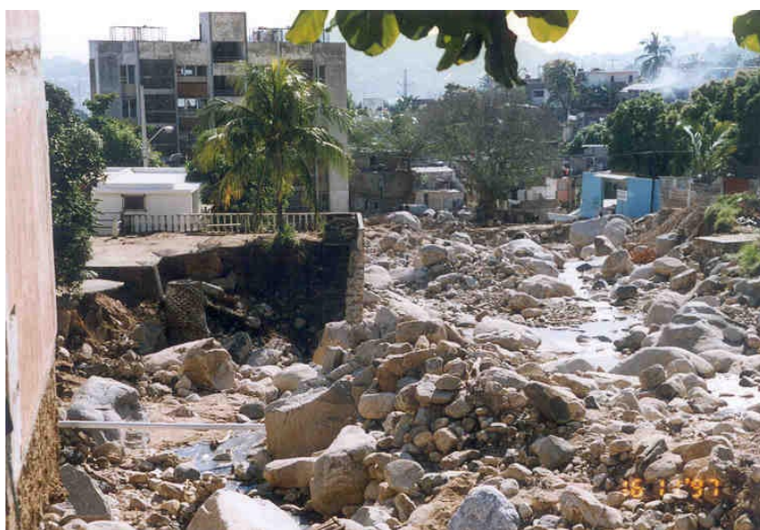
Figure 8. Devastations by a broken out torrent; destroyed culvert on the left, former street on the right side; side retaining wall of the inlet collapsed, street deeply eroded and destroyed.
