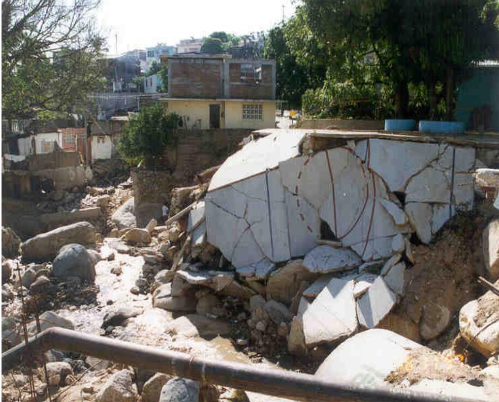
Figure 6. The former street in the center is completely washed away, the basketball field to the right was undercut and collapsed.
